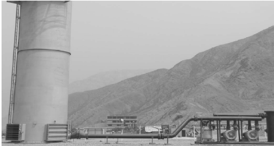
Picture (3) Huaycoloro landfill gas recovery facility Source: Petramas, 2007
